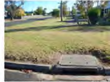
5 Lack of provision for people with disabilities
