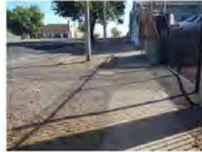
2 Missing links in the footpath network
