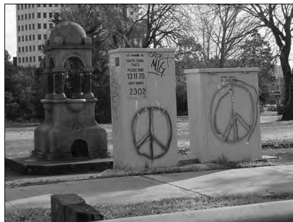
Inappropriate placement of modern services close to Contributory Elements of a Heritage Place
