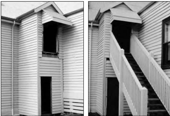
Reconstruction of the rear stairwell of the Toongabbie Mechanics Institute – before (left) and after reinstatement of missing parts (right)
